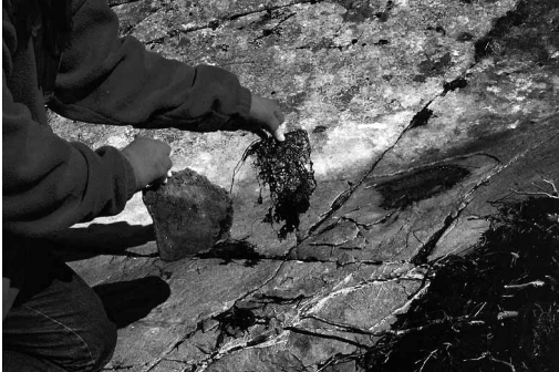
Fig. 3. Unsuccessful experiment with gluing loose exfoliation crusts at Vingen, Bremanger, W. Norway, by use of a glue containing Mowilith. The crust has loosened and a whitish-glossy layer of hardened glue is visible in lower part of the picture. The cracking effects of thin herbaceous roots are also visible. Photo (1997) S. Bakkevig.
