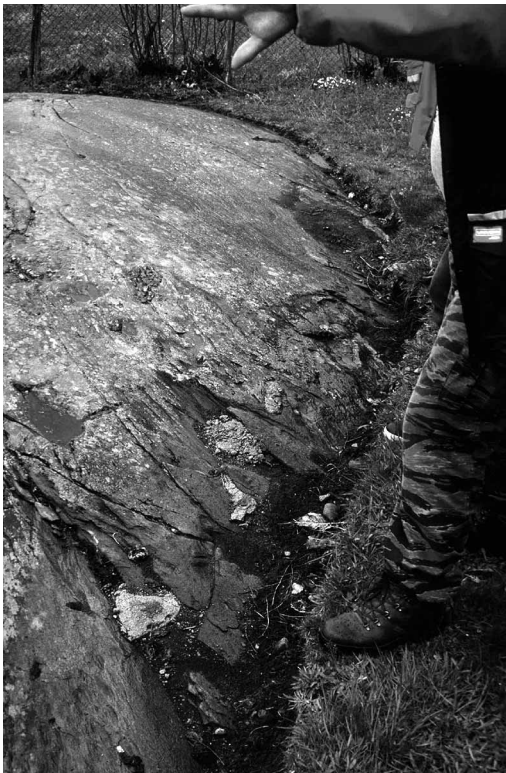
Fig. 4. Unsuccessful use of mortar on the rock art site Bakke I, Jondal, Hordaland, W. Norway. The mortar has begun shrinking and cracking in less than 20 years. Photo (1998) S. Bakkevig.
