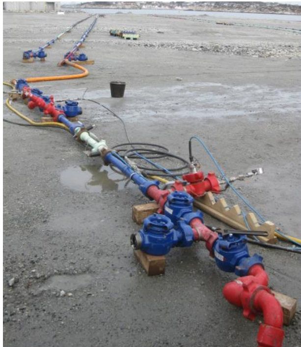
Figure 5: Test loops and connections out of pumps
