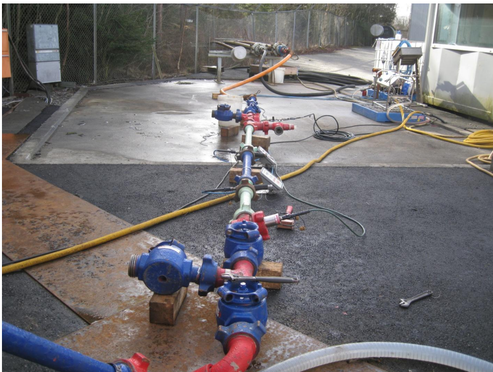
Appendix 15: Double block and bleed, flow meter, pressure gauge and PSV set up IRIS test yard
