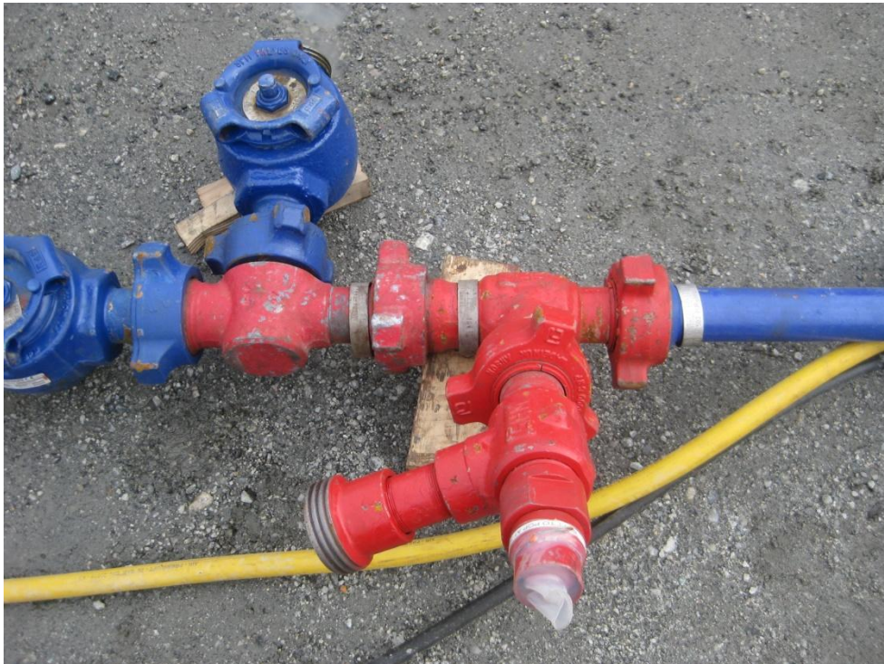
Appendix 11: Pressure safety valve (PSV) at test site
