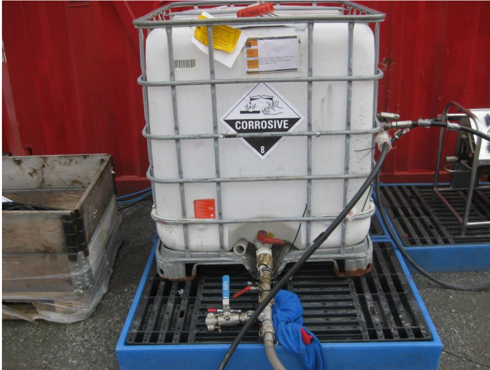
Appendix 5: Chemical tank (Xlinker tank)
