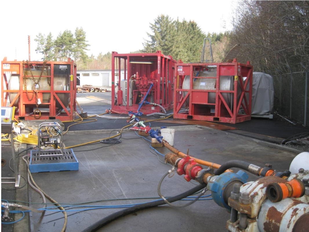
Appendix 14: Experimental set up at IRIS test yard
