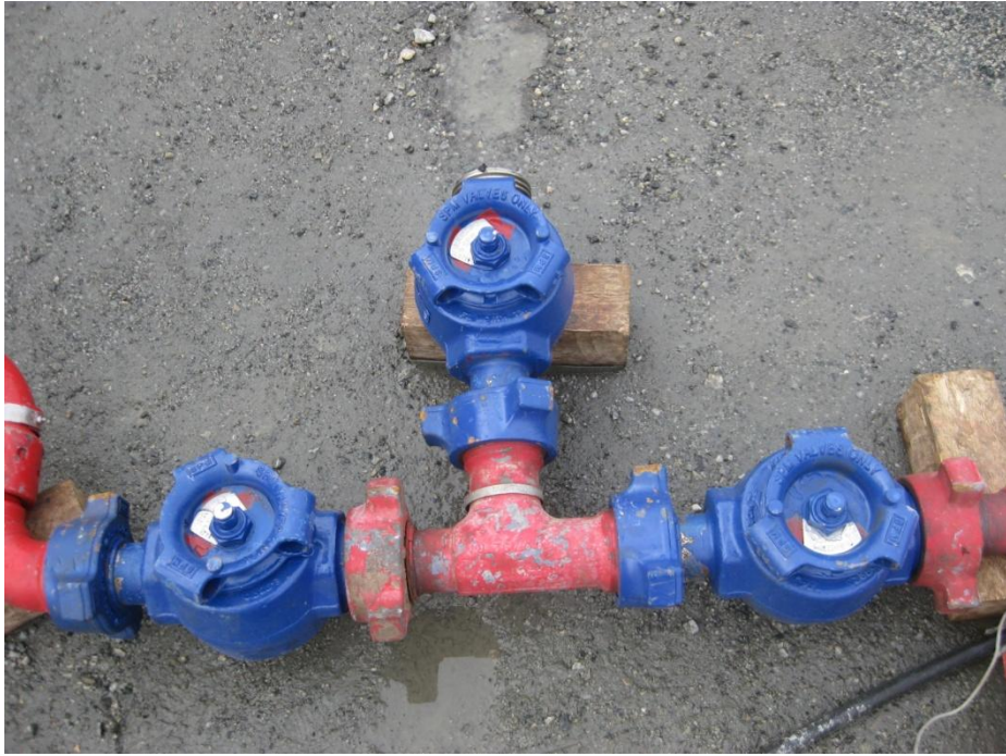
Appendix 12: Double block and bleed valve at test site
