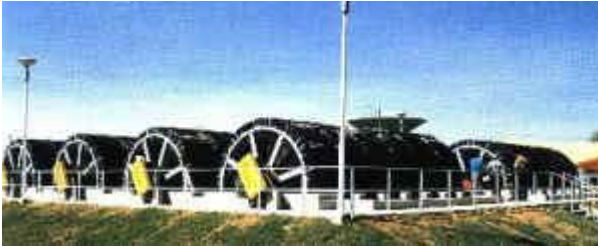
Fig. 1.3.9. Large RBC installation. Multiple installation of 3.66 m diameter RBC's at a plant serving 50,000 people. (From www.keepprocess.com )
