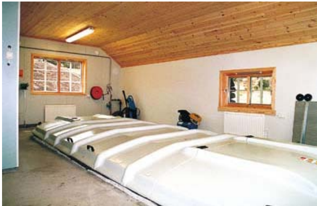
Fig. 1.3.8. RBC Housing inside. BK NuDisc – Preikestolhytten, Norway. This plant serves a Youth Hostel and Restaurant with the load fluctuating considerably through the year. The effluent quality requirements are stringent; nutrient removal is required with total phosphorus to be reduced to less than 1ppm. The plant is housed in a high class building to provide easy access for maintenance in Arctic Scandinavian weather conditions. ( http://www.keeprocess.com/SL007-RBC.pdf )
