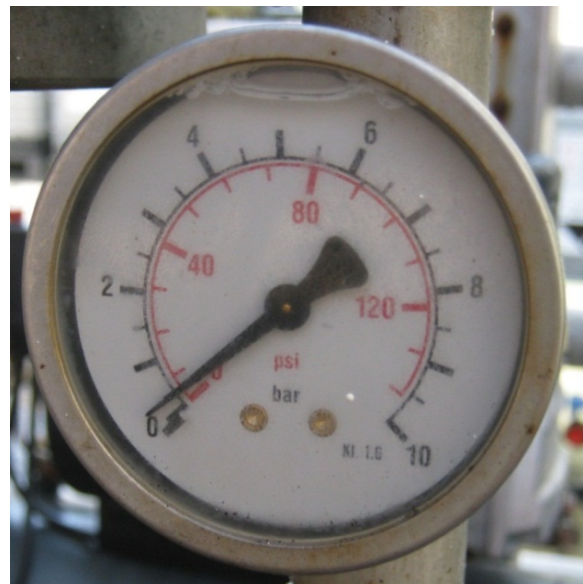
Figure 5.6 Pressure indicator at the cyclone
