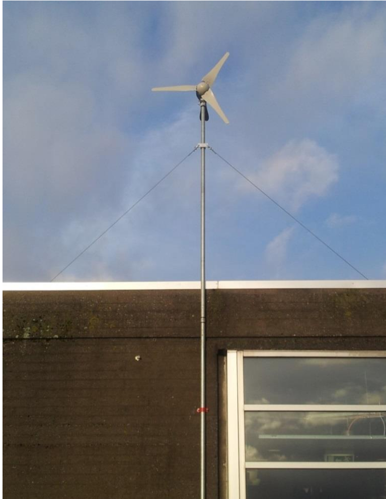
Figure 2.3: Installed Coleman 600W wind turbine.
