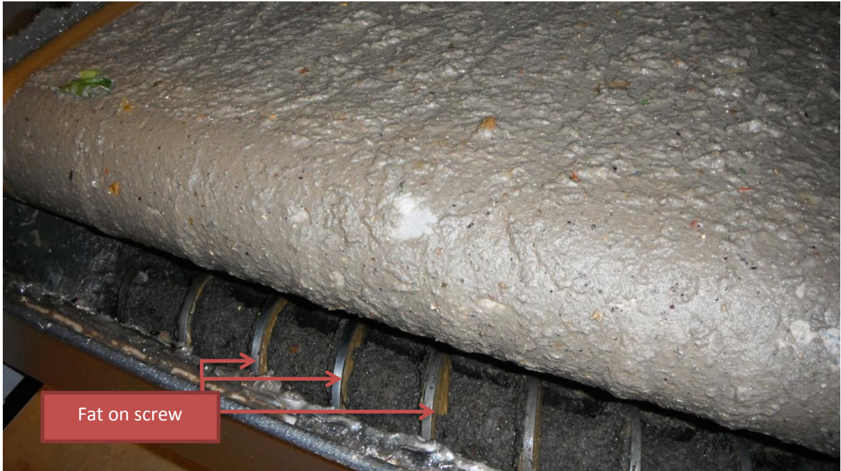
Figure 4: Salsnes Filter SF6000 with waste attached before airknife. Note that toilet paper is visible on the filter, and fats are visible on the screw.
