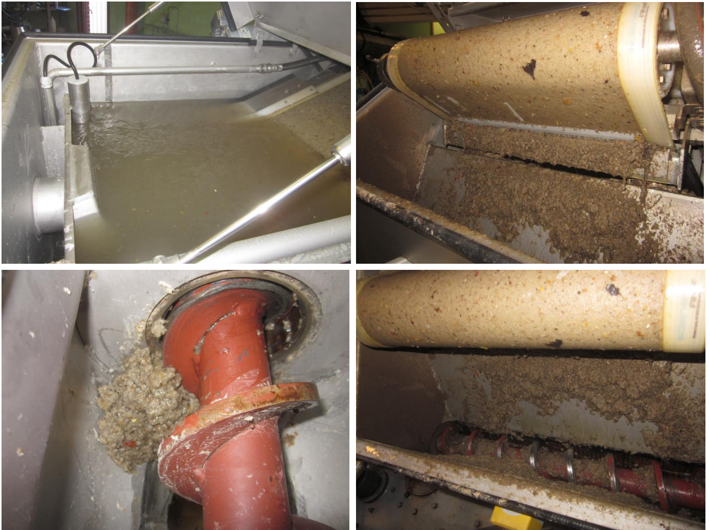
Figure 12: Clockwise from top left: 1. Wastewater influent being filtered. 2. Solids being blown off into trough by air knife. 3. Solids being transported out of trough via screw. 4. Solids exiting the filter (normally where the dewatering unit is attached).
