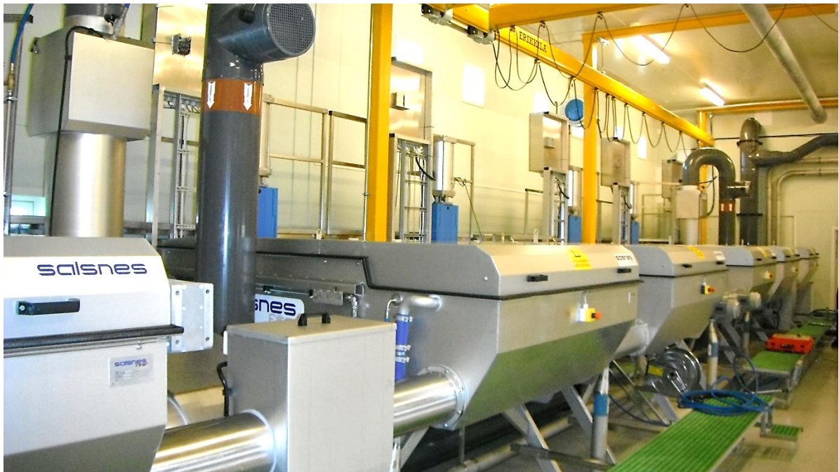
Figure 1: Salsnes SF6000s at Tiendeholmen Renseanlegg in Namsos, Norway.
