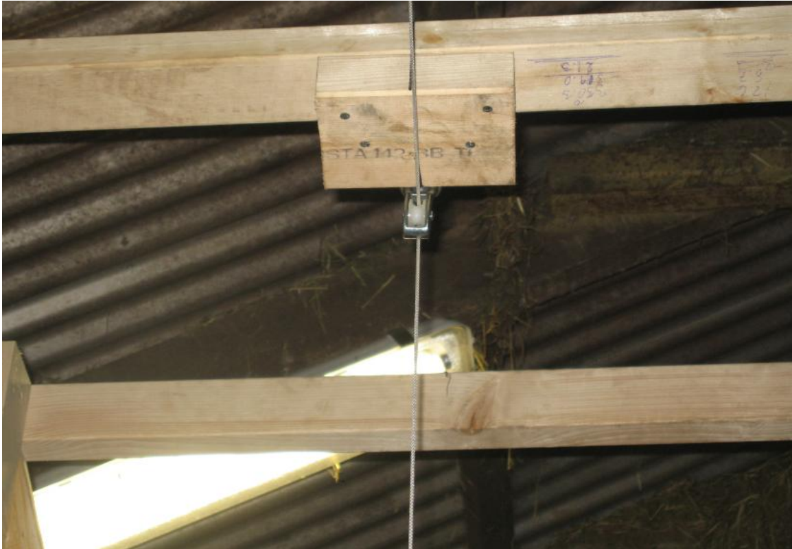
Figure 15a. Pulley for the wire which was used to apply tension force to the pipeline.
