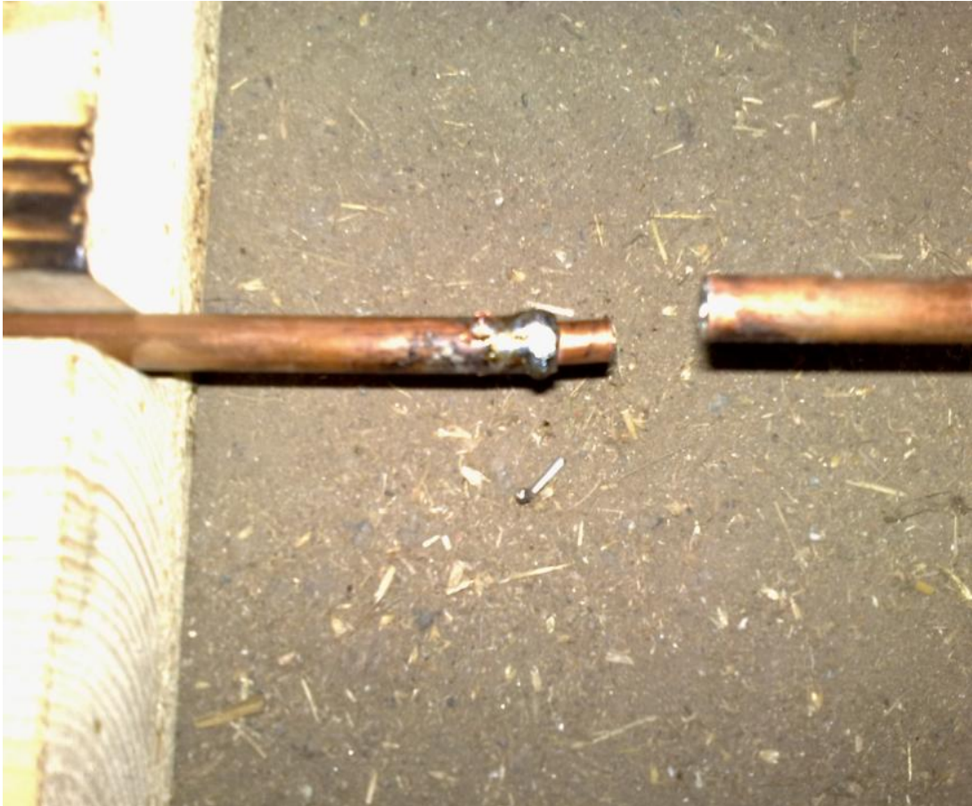
Figure 11. A piece of a smaller diameter pipeline was inserted into the main pipeline before soldering
