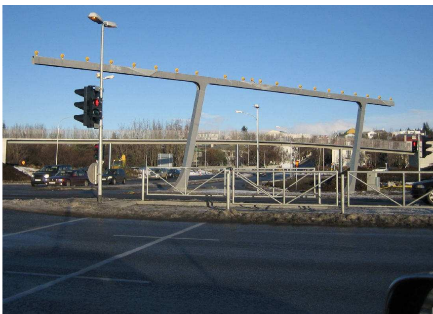
Figure 3.1: The mast supporting flight control lamps. Large oscillations were observed at the cantilever beam shortly after installation [Bessason and Snaebjörnsson, 2008].
