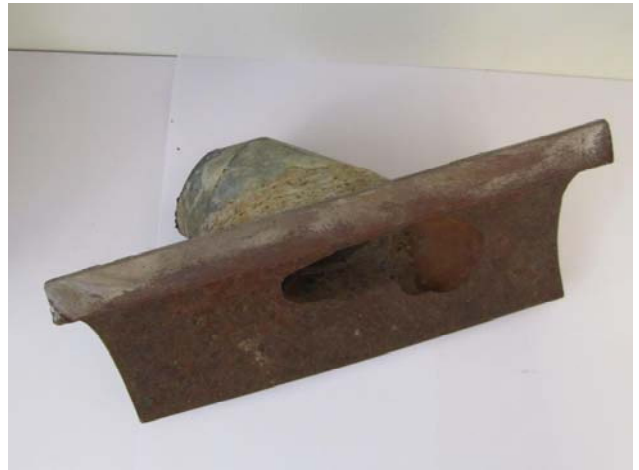
Figure 2.9: Corrosion at the point that chemicals are injected to the pipe
