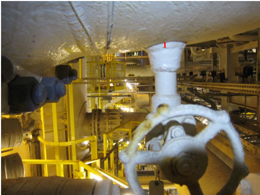
Figure 2.10: welded valve to a pipe, difficult to inspect
