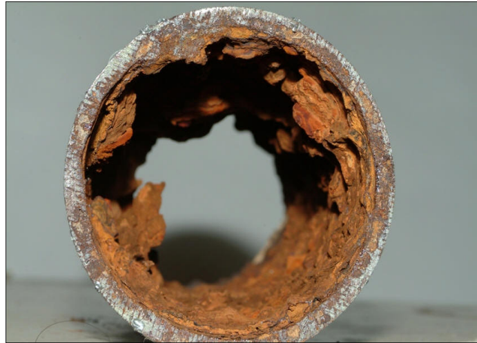
Figure 6.6: MIC in wet fire sprinkler system (Source: http://www.stroudsystems.com/pm_fss.html )
