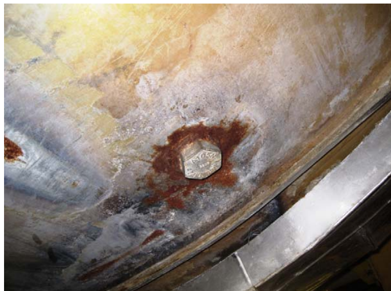
Figure 6.2: Galvanic corrosion of a tank
