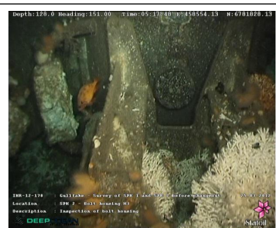
Figure 4.19: Behind bolt housing with flange
