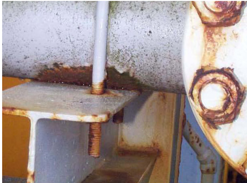
Figure 20. Progressive paint destruction (Britton, 2002)
