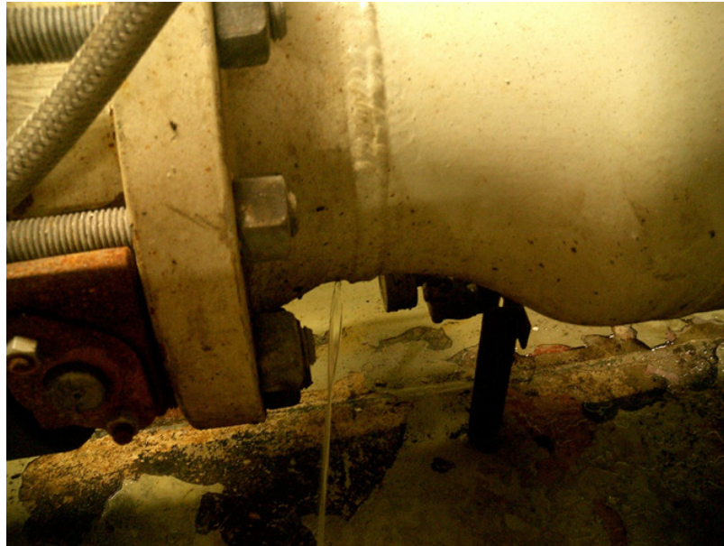
Figure 28. Leakage in a CS pipe
