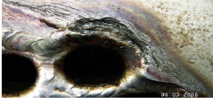
Figure 26. Crevice corrosion in seawater cooler finally leading to leakages. (Heselmans ,2006)
