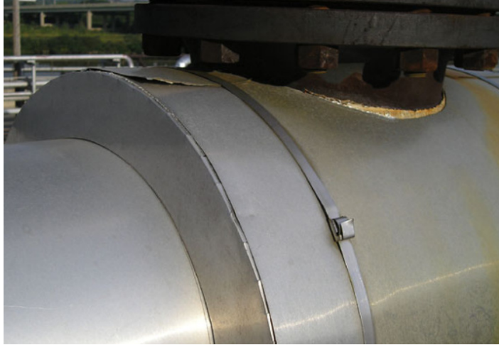
Figure 7. Absence of final barrier on jacketing (Lettich, 2007).
