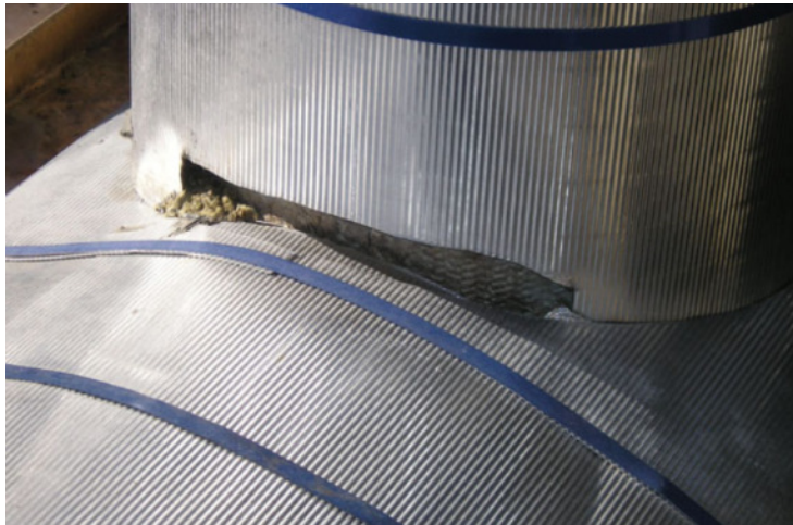
Figure 8. Improper installation of jacketing (Lettich, 2007).
