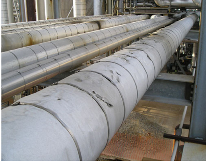
Figure 11. Small holes in the weather barrier (Lettich, 2007).
