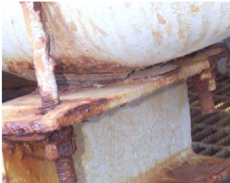
Figure 21. Advanced crevice corrosion (Britton, 2002)
