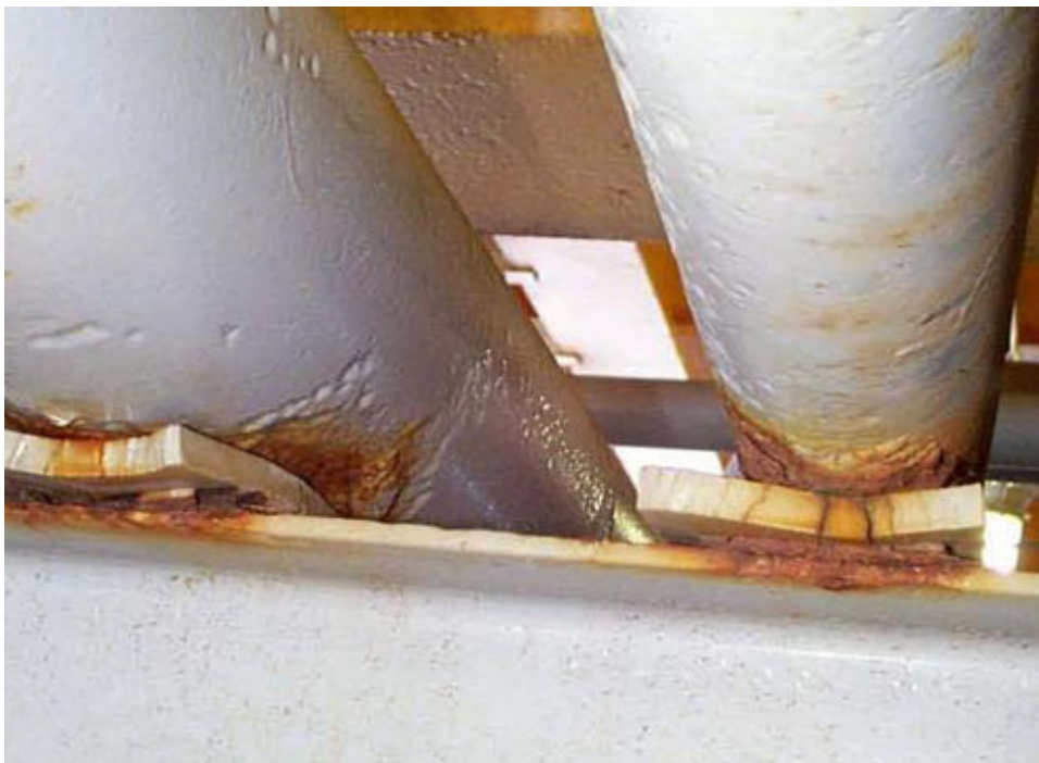
Figure 22. Rubber pads accelerate crevice corrosion (Britton, 2002)
