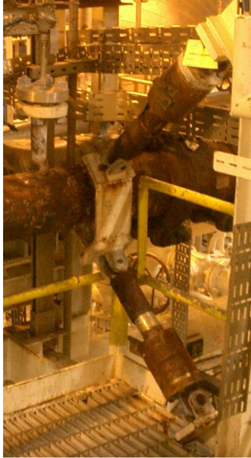
Figure 24. Corroded snubbers and pipe after insulation removal in the process area with high humidity due to, among other things, leaking roof
