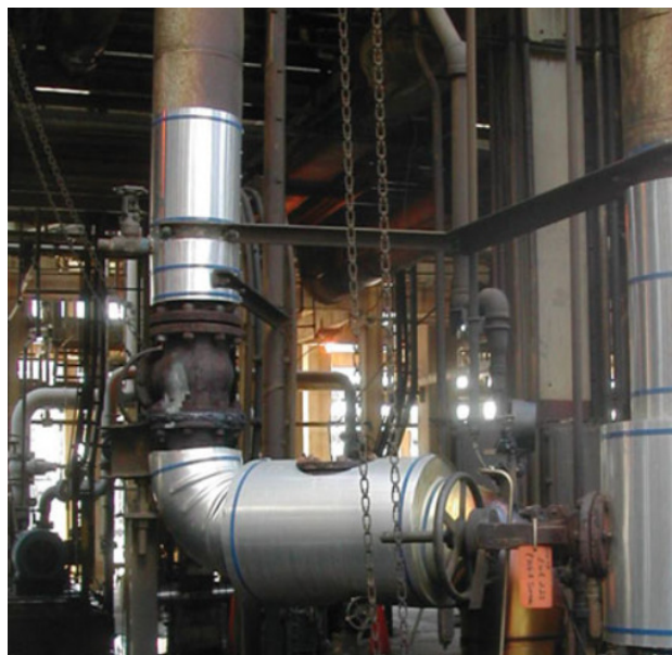
Figure 9. Lower sections of the jacketing are installed over the top of upper section leading to water ingress (Lettich, 2007).
