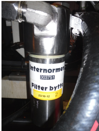
Figure 9-21 HPU Filter housing
