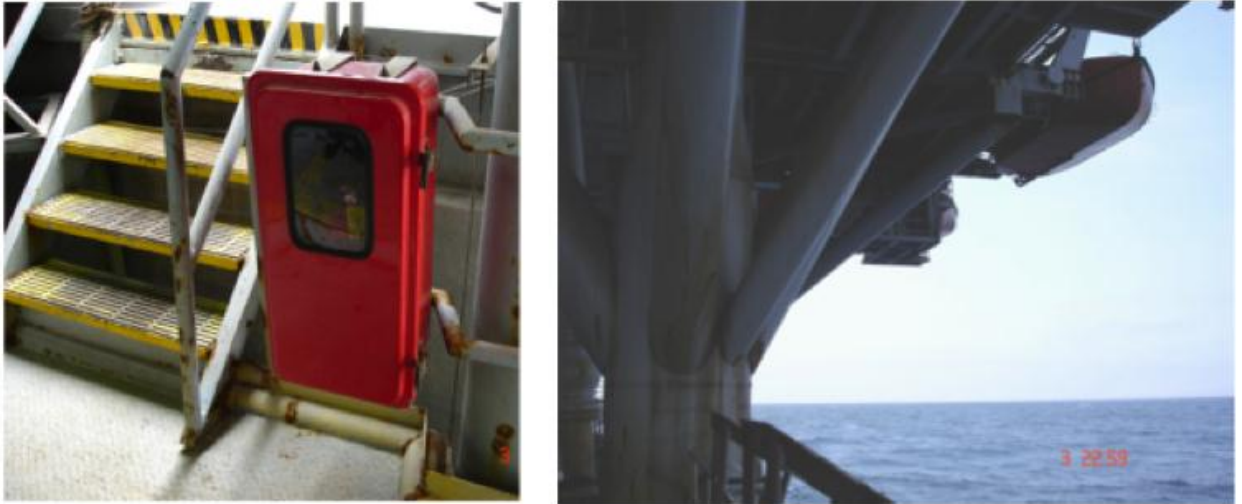
Fig. 40 Fire extinguisher and life rafts [19]
