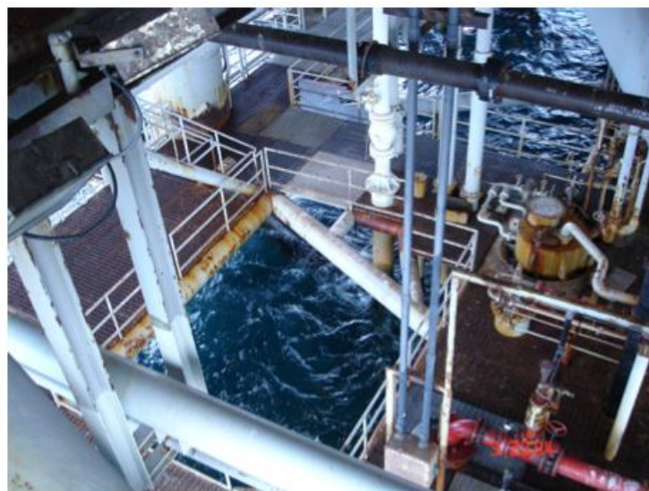
Fig. 42 Valves and deck of a Jack-up rig [19]
