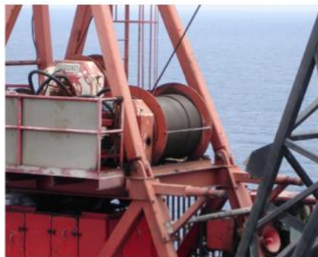
Fig 43. Unprotected cables ice readily and they may become inoperable [19]
