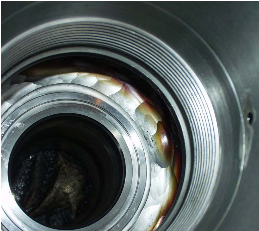
Figure 5-8 Erosion in choke valve (AkerSolutions database)
