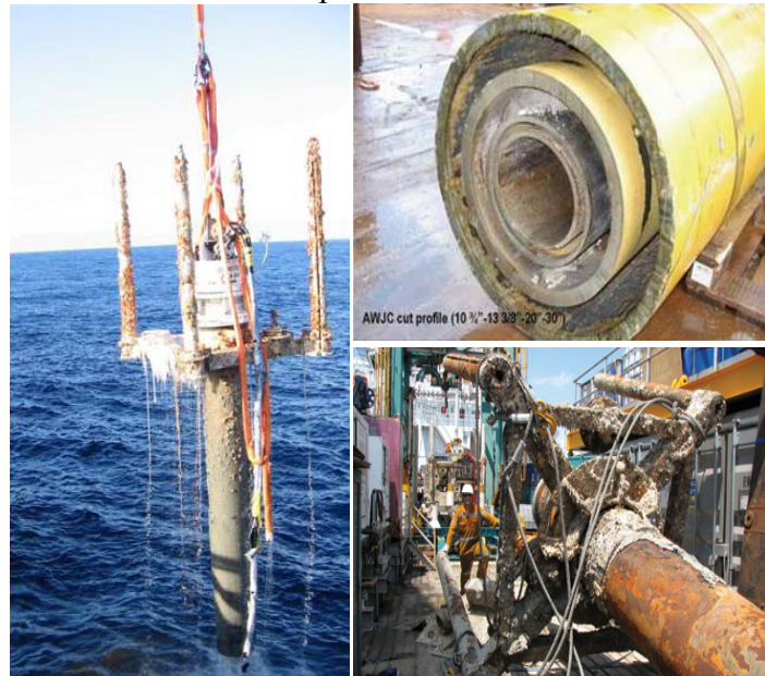
Figure 10. Severed casing-strings and WH pick up.
