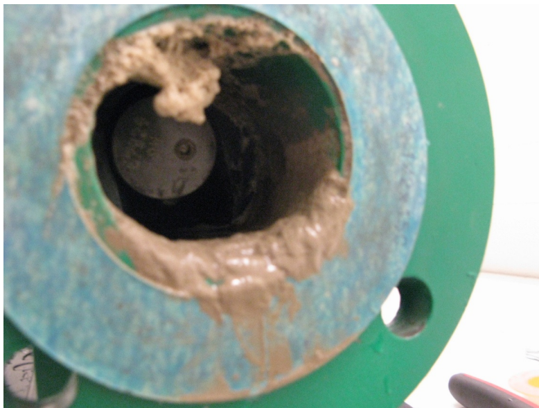
Figure 21: Outlet of pump after repeated water flushing.
