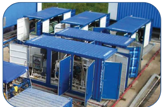
Fig. 20 Nitrogen Generation Unit (Ref. no 34.)
