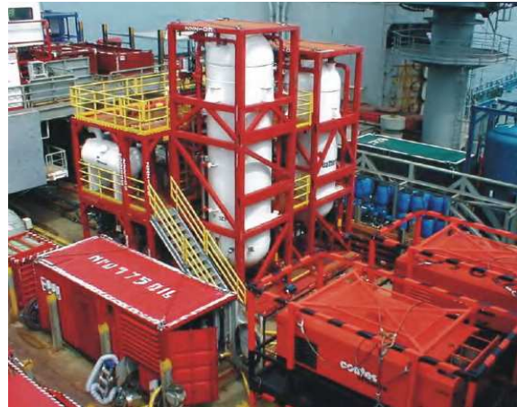
Fig. 21 MPD Multiphase Separation System (Ref. no 34.)
