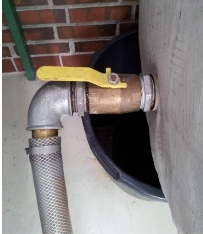
Water tank valve open.
