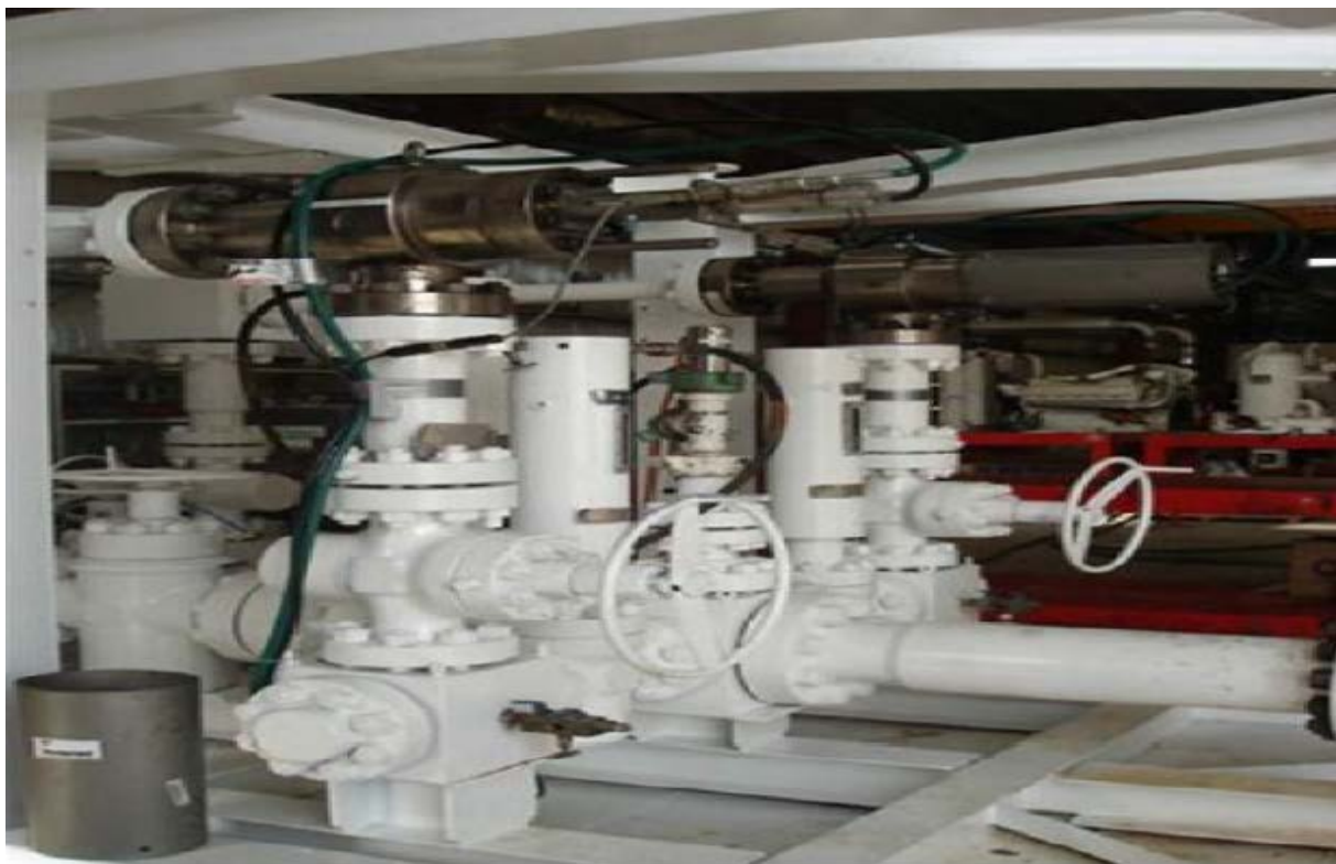
Figure 17: Semi-Automatic Choke Manifold [21]
