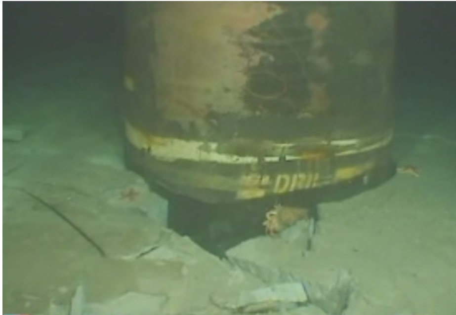
Figure 40 Conductor cement 12 days after the grouting job [71]
