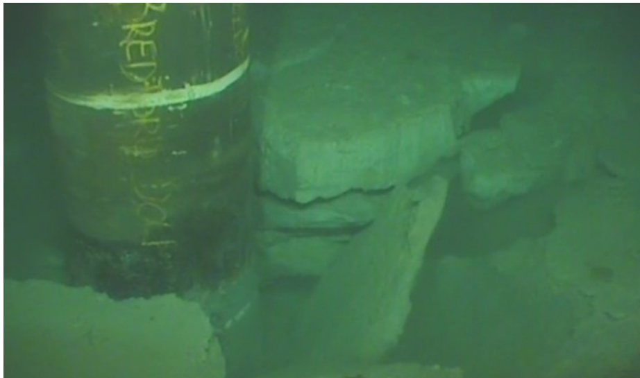
Figure 38 ROV image showing the first conductor cement failure [71]
