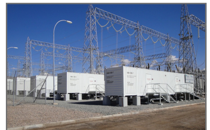
Dynamic energy solutions for a smarter grid
