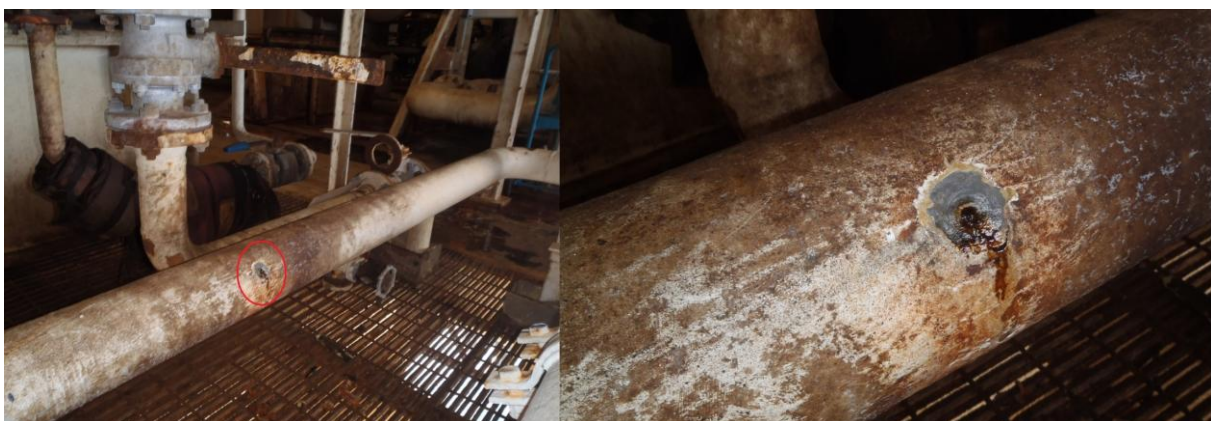
Figure 21: Internal MIC failure (from an undisclosed operator in the North Sea)
