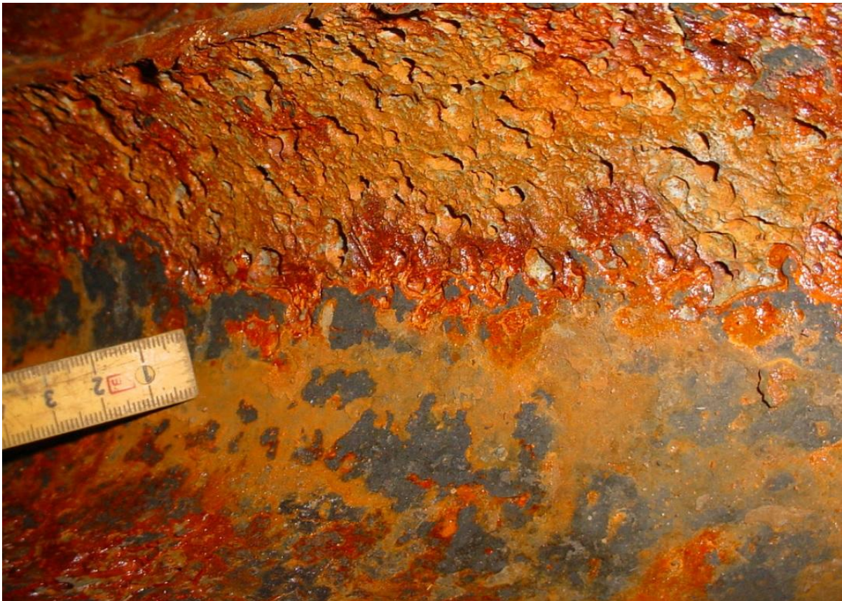
Figure 2: Pitting corrosion caused by MIC. (Obtained from an undisclosed operator in the North Sea)
