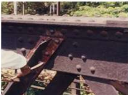
Figure 40 Some of corroded location of the bridge [30]
