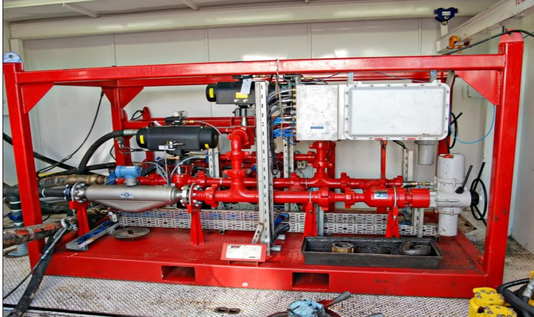
Figure 2.5: Flow Control Unit [5]
