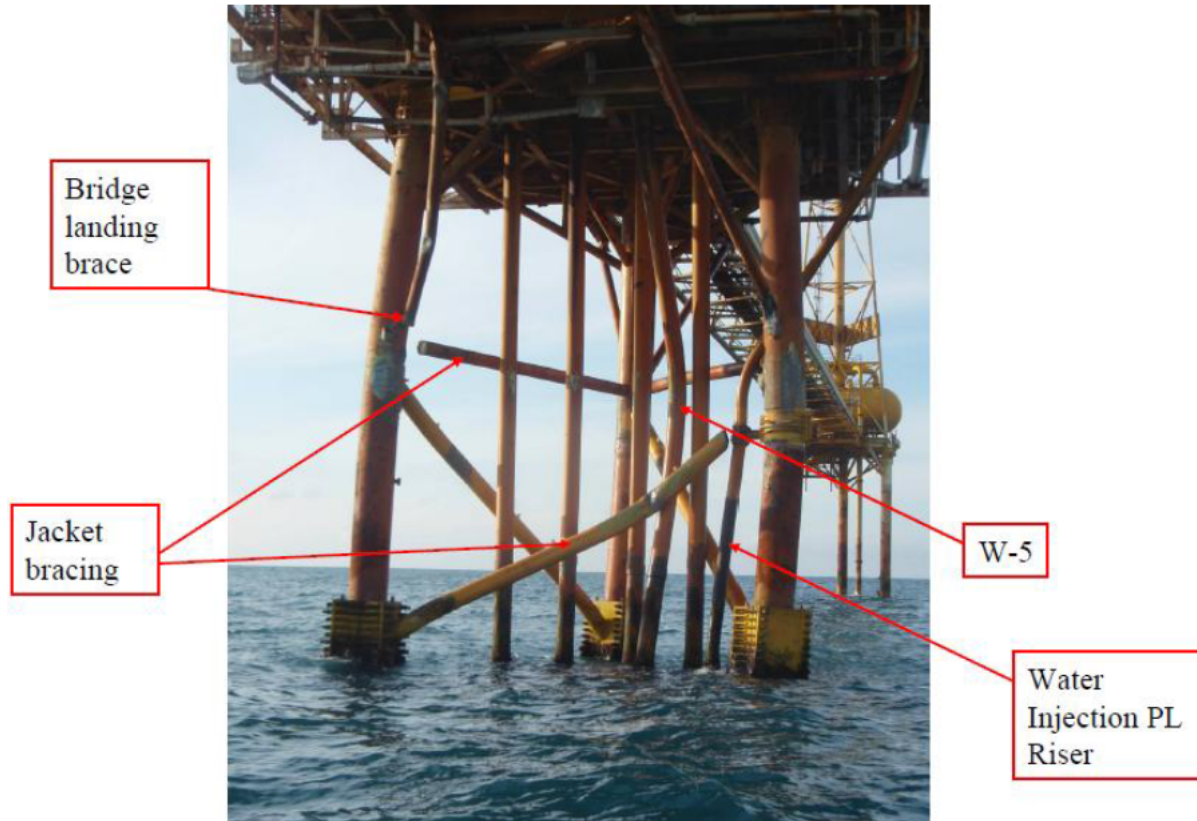
Figure 1-2 – Damage on Ekofisk 2/4-W platform (Ref. /19)
