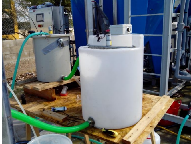
Figure 3.7: 20 Liter tank in combination with a 50 Liter Pilot Scale Tank Flocculator configuration 2.
