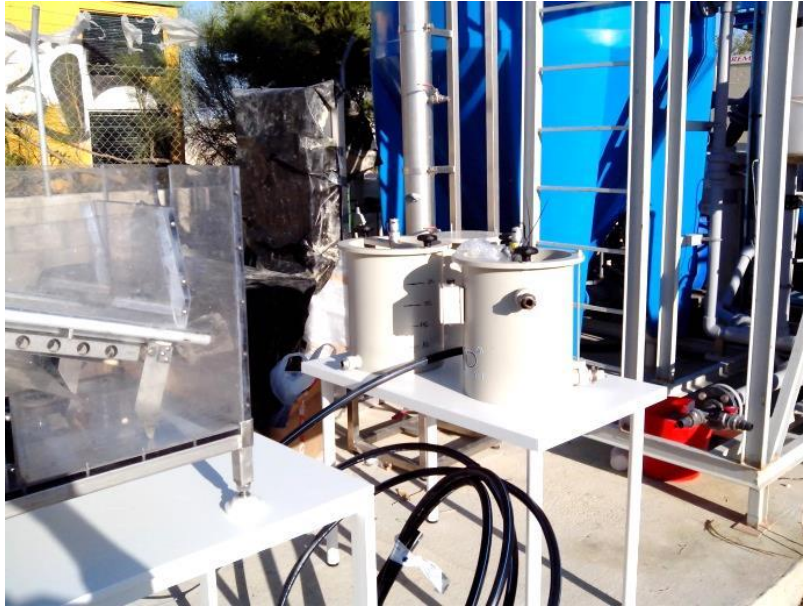
Figure 3.5: Pilot scale tank flocculator configuration provided by Asio®.
