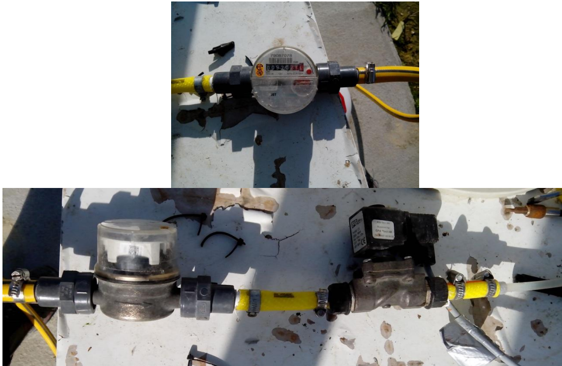
Figure 3.20 Up: Flow meter. Down: Flow meter and solenoid valve connected to each other.
