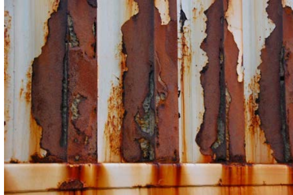
Figure 22. Deterioration of blast wall connections(Stacey, 2010)
