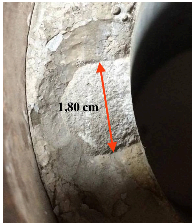
Figure 62: The damaged caused by the reflected spark.
