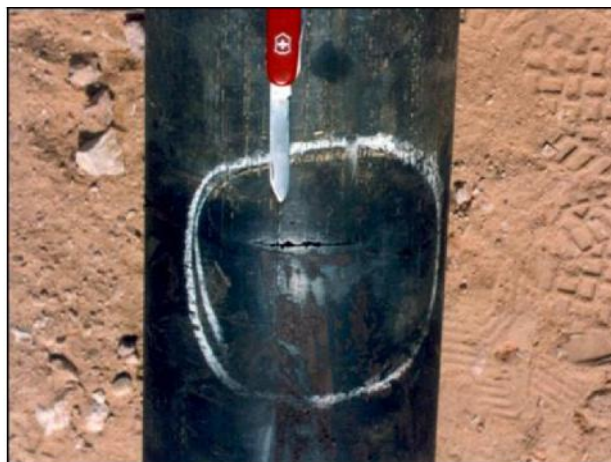
Figure 10: Crack that developed due to bending fatigue from backward whirl ( Internal Document - Dynamic
