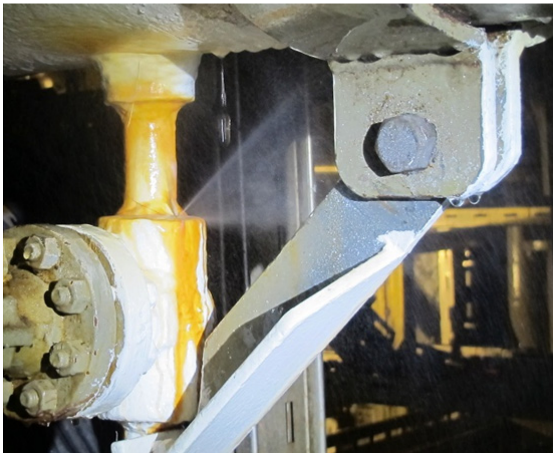
Figure 22 - Example of leak on a weld (Courtesy of Aker Solutions MMO)
