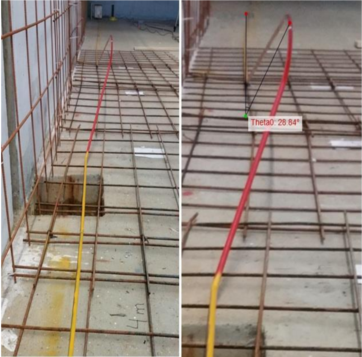
Figure F9- for test 15, See Section 7.5.2 for installation parameters.
