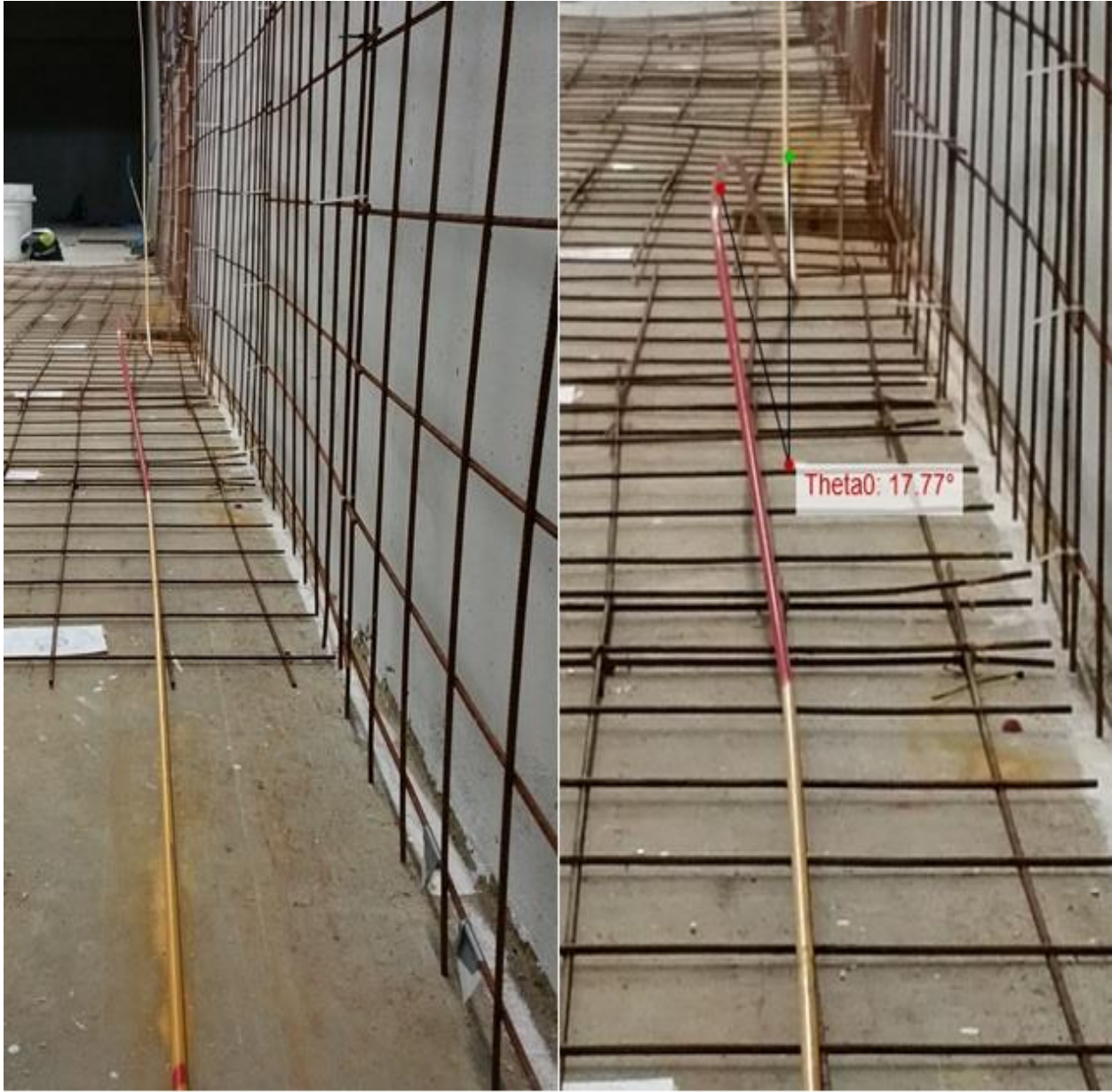
Figure F7- for test 12, See Section 7.4.2 for installation parameters.
