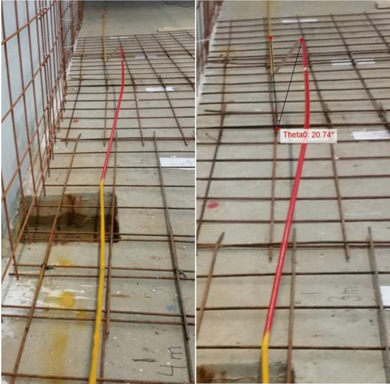
Figure F10- for test 17, See Section 7.6.2 for installation parameters.
