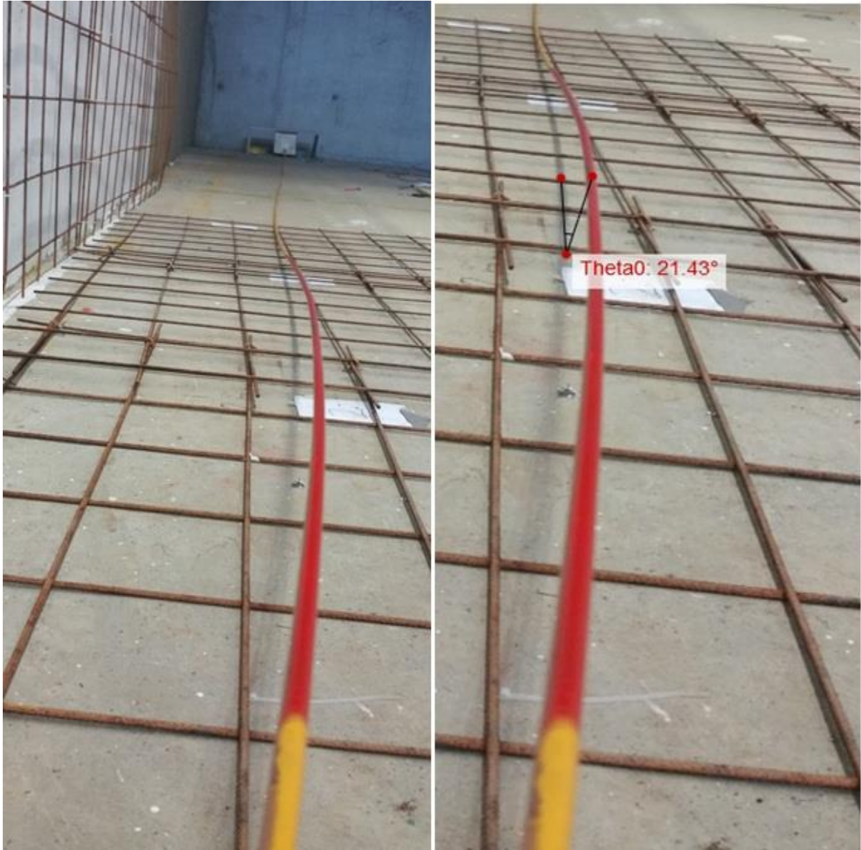
Figure F4- for test 6, See Section 7.3.6 for installation parameters.
