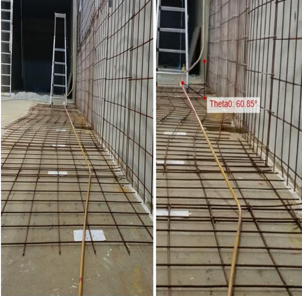
Figure F-1 for test 3, See Section 7.3.3 for installation parameters.
