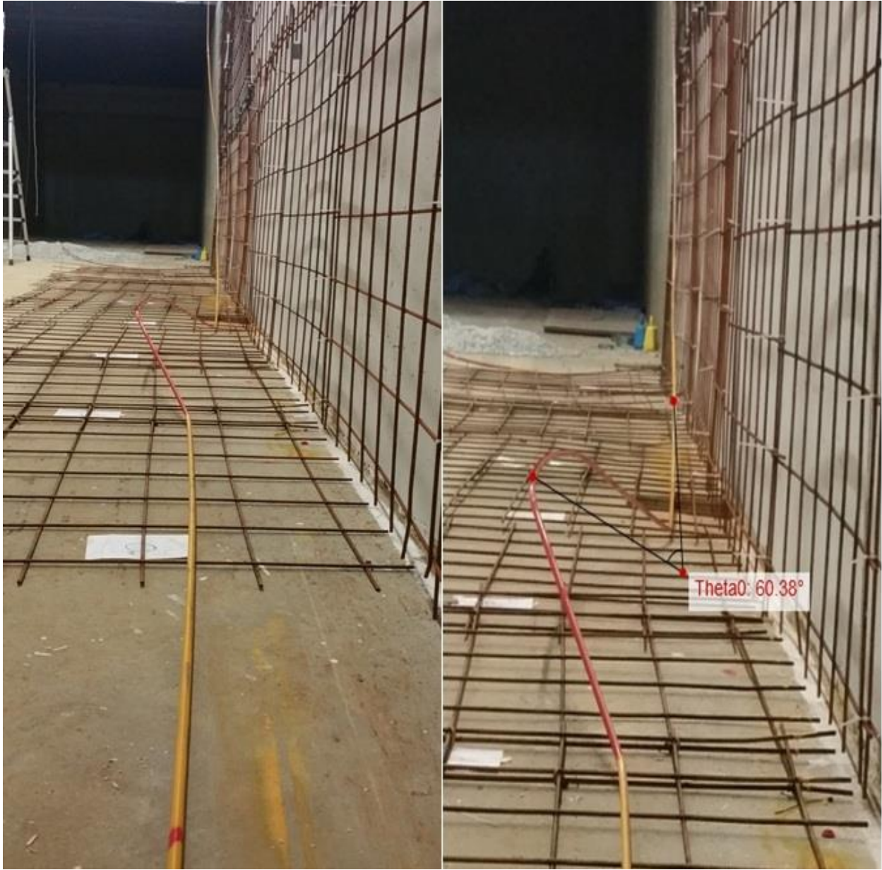
Figure F6- for test 9, See Section 7.3.9 for installation parameters.
