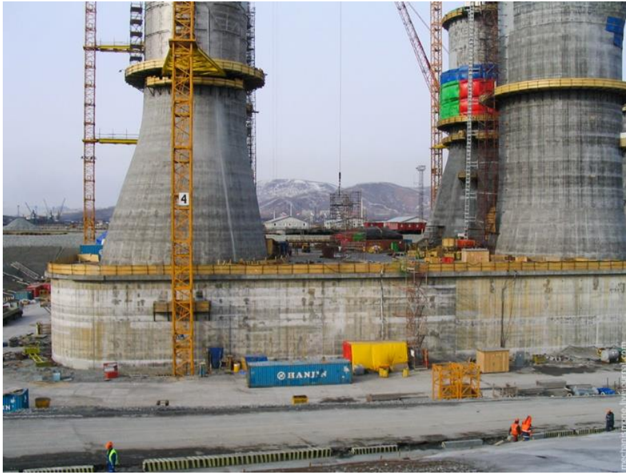
Figure 48. Construction of the Lun-A concrete GBS at the Wrangel site, Vostochny Port (Photo courtesy of Sakhalin Energy Investment Company)
