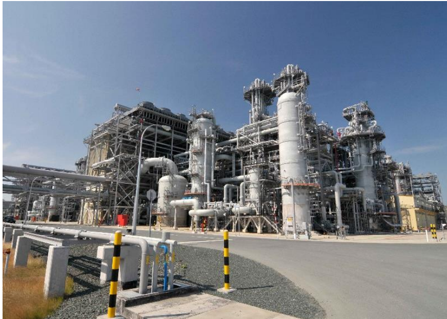
Figure 19. Prigorodnoye Production Facility of Sakhalin-II project (Photo courtesy of Sakhalin Energy Investment Company Ltd.)
