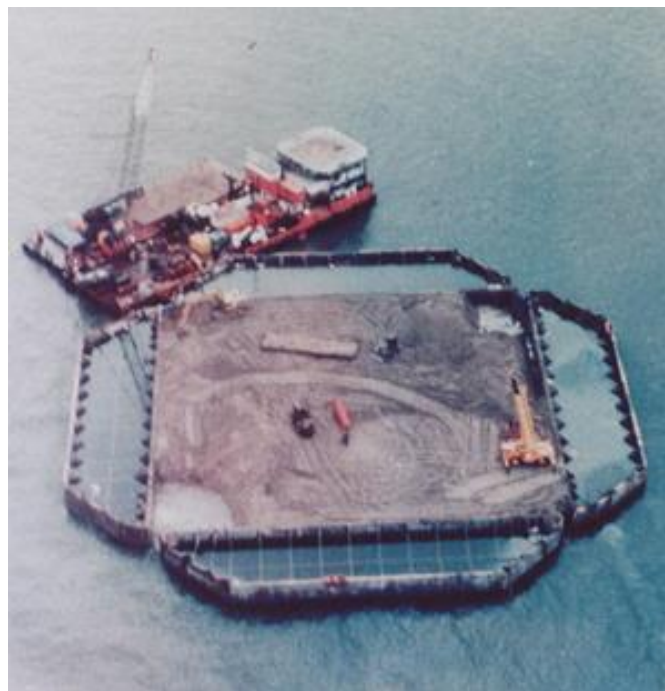
Figure 36. Dome's Tarsuit Caisson Retained Island in the Canadian Beaufort Sea - Under Construction
