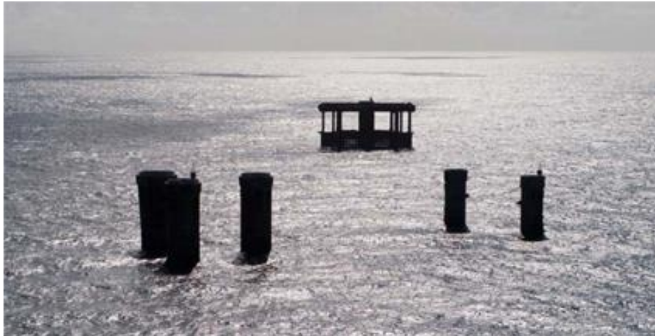
Figure 50. Remaining concrete structures at the Frig Field Center, North Sea (photo: Norwegian Petroleum Directorate)
