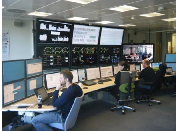
Figure 3.11 Valhall Onshore Control Room
