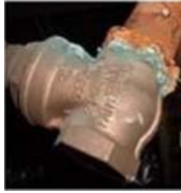
Figure 4.3: Galvanic Corrosion of Dissimilar Metals, More Anodic Metal Corrodes
