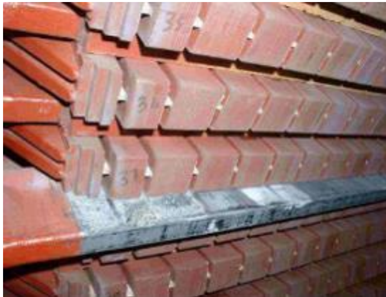
Figure 29: Abrasion caused by loose coil in slot. Image source: JIP project.
