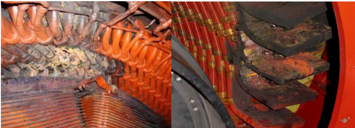
Figure 2: Catastrophic failures due to burnt windings. Image source: JIP project.
