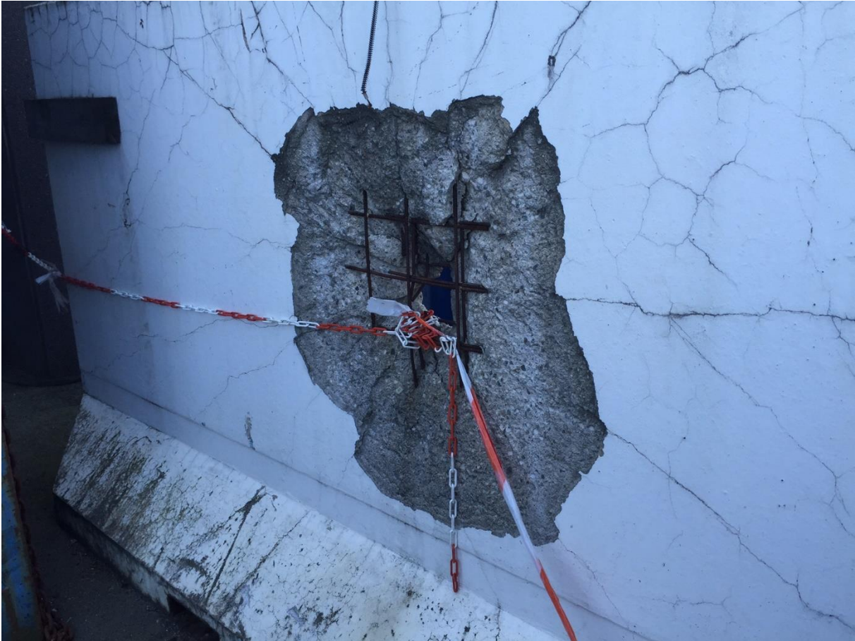
Figure 26 Scabbing of safety wall
