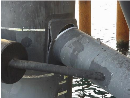
(A) Fatigue through crack
