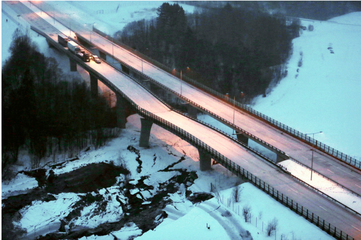
Figure 2.6: Quick clay landslide collapsing the bridge at Vestfold, Norway ( www.vg.no )
