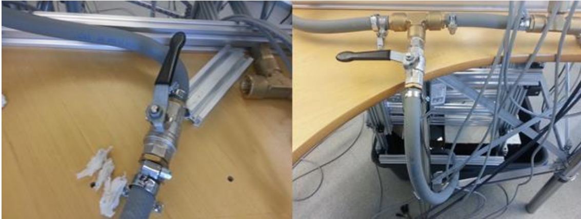
FIGURE 32 - OBSTRUCTION VALVE(LEFT), LEAK VALVE(RIGHT)
