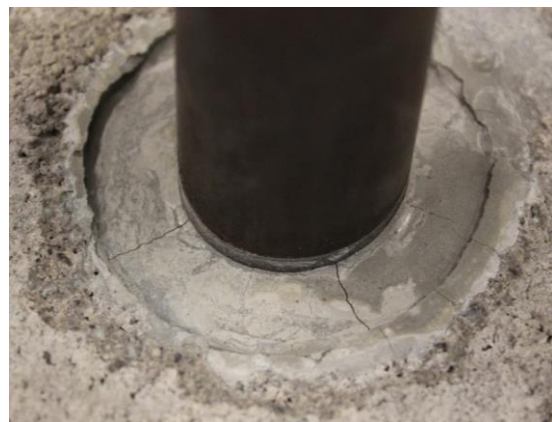
Figure 4.61: After one temperature cycle the cement had fractured due to heating and expansion of the casing.
