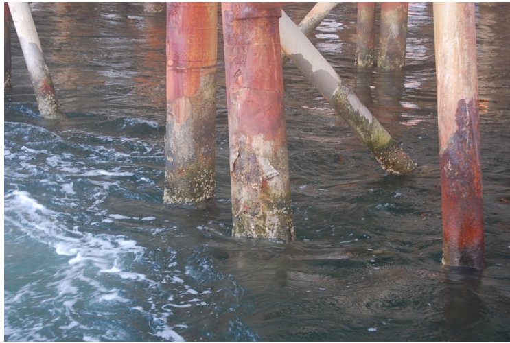
Figure 2.4: Example of corrosion near the splash-zone [21]
