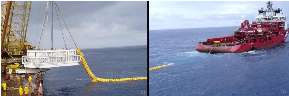
Figure 1-4: Left: Dummy manifold being lowered into the water. Right: The Installation vessel, an AHTS
