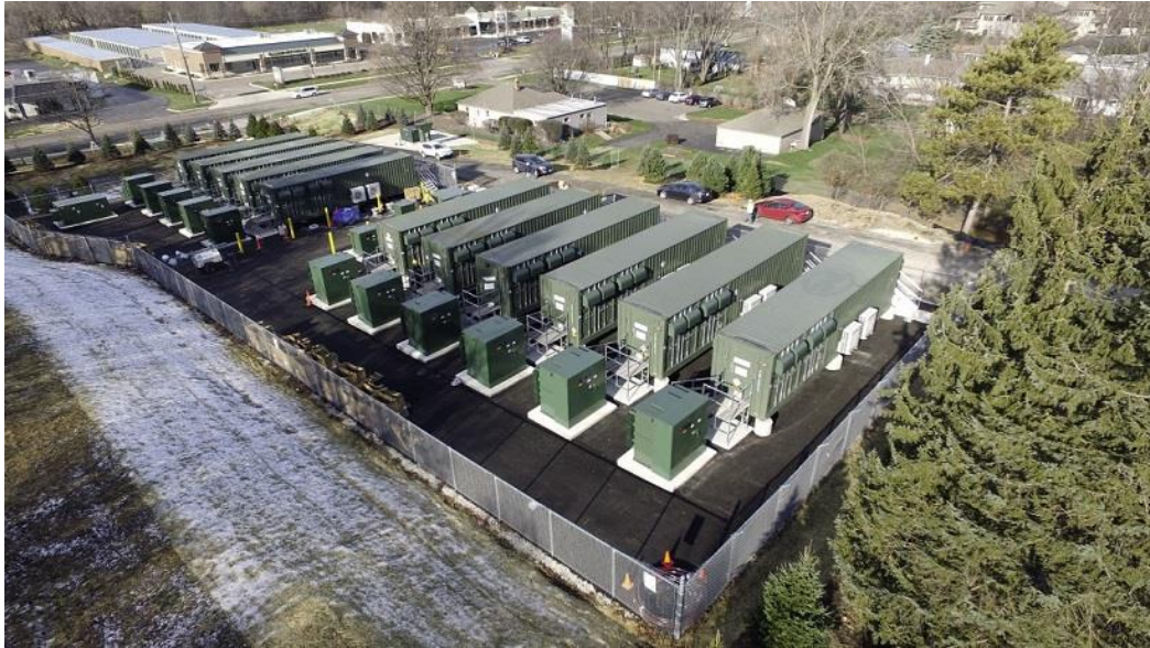
Figure 15 500 MW battery facility. (ROSELUND).
