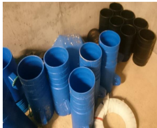
Figure 49 - Spare Parts inside of the barge
