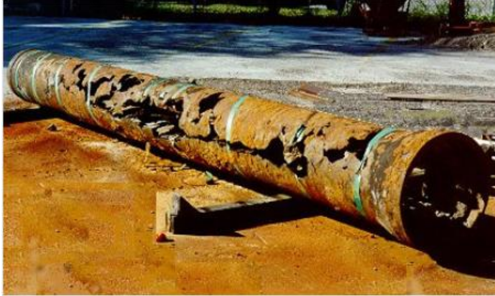
Figure 2.1 Impact of corrosion in the pipelines (Engineers)
