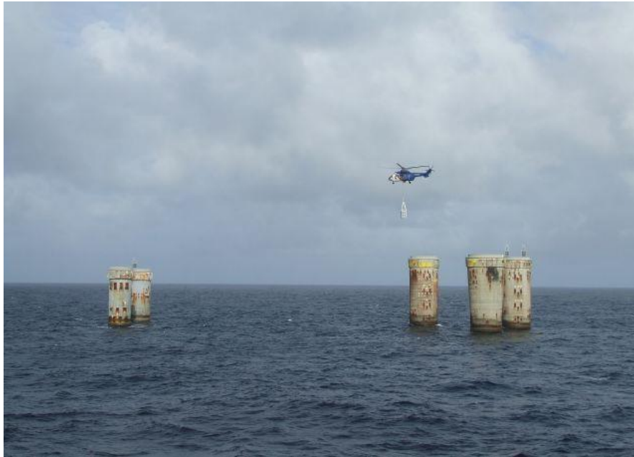
Figure 18: Installation of AtoN on the concrete legs left behind after the decommissioning of Frigg [35]
