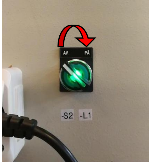
Figure 16 Secondary fuse box switch
