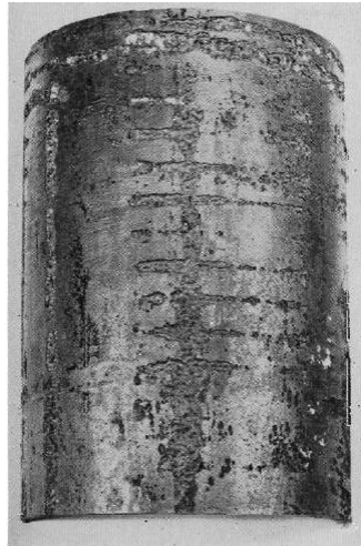
Figure 15. H 2 S pitting corrosion due to bacteria metabolism on external part of casing [21]
