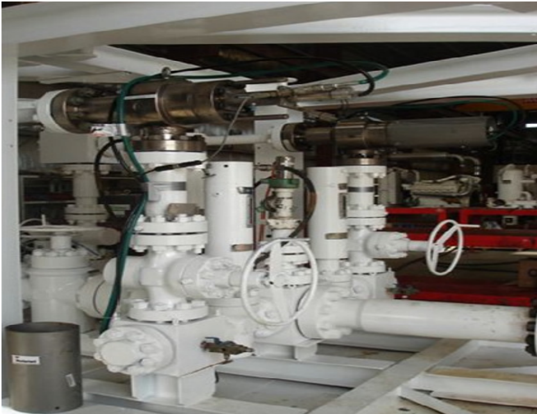
Fig 18: Semi Automatic Choke Manifold [23]
